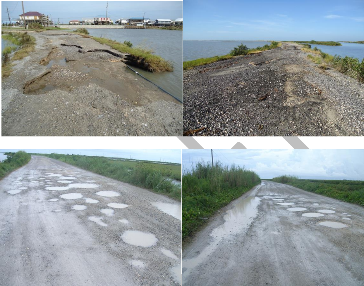
Elmer's Access Road - storm damage and routine "wear and tear"
