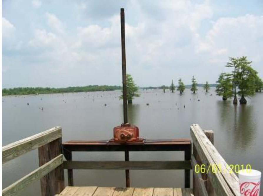
Figure 3. Water control structure located at the dam on the southern end of Turkey Creek Lake, LA.
