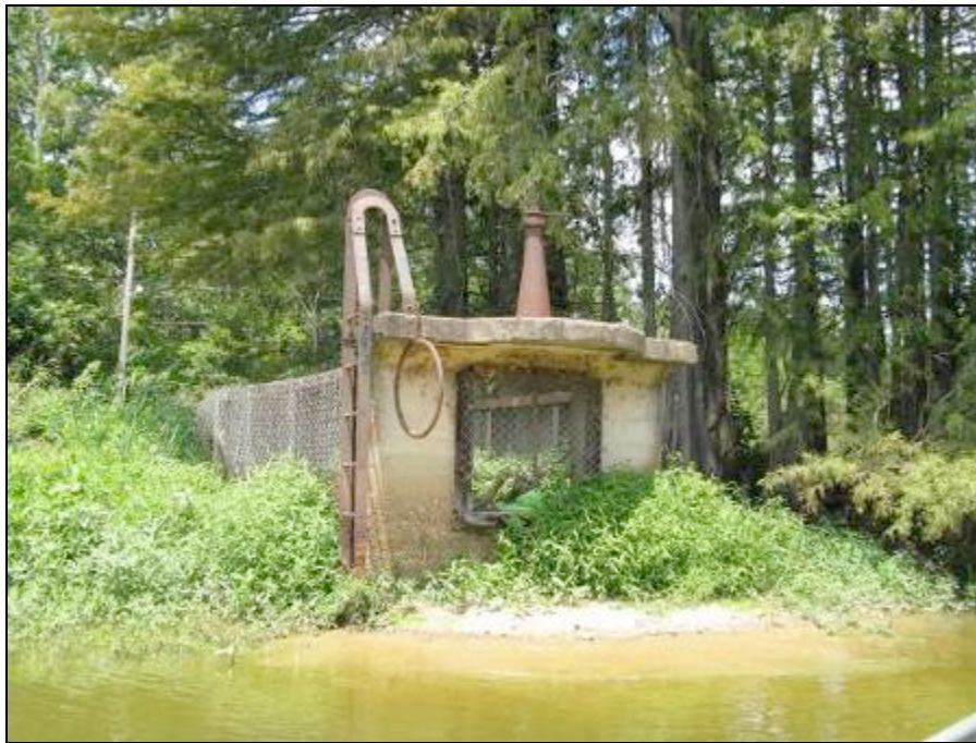
Figure 1. Horseshoe Lake control structure at 2.5 ft. below pool stage.
