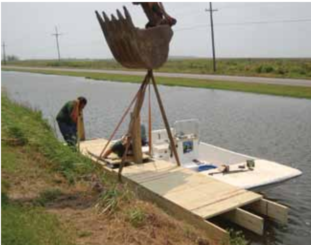
Coastal Operations staff building dock for Terrebonne Aquatic Clinic on Bayou Pointe-aux-Chenes.
