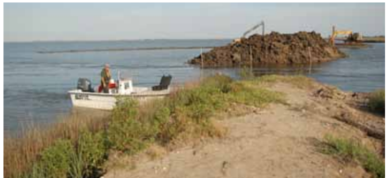
Pictures of the breach in the Pointe-aux-Chenes/DU Management Unit prior to and during repair.
