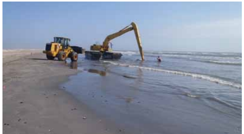
The image above is of mechanical treatment occurring on Elmer's Island during November 2011. The long reach excavator was used to remove oil mats found in the surf zone.
