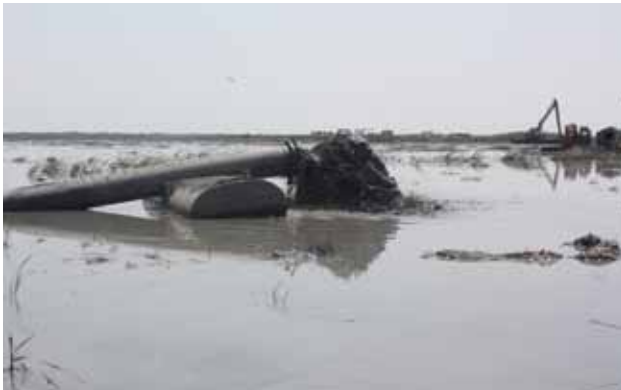
Dredge Disposal as part of the East Marsh Island Marsh Creation Project.
