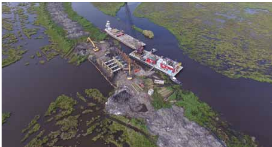
This four-pipe water control structure, located on the southeastern portion of the refuge, is one of a network of water control along the southern Mermentau Basin.
