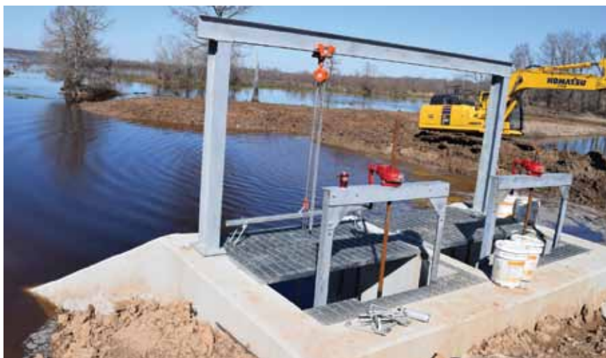
New water control structure at Wham Brake.
