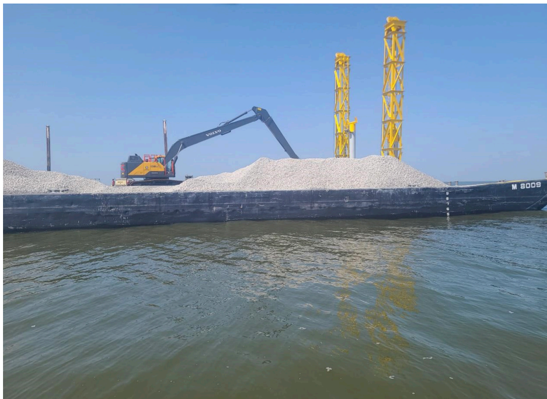
EXCAVATOR DISPERSING LIMESTONE FOR THE CONSTRUCTION OF THE 2022 DRUM BAY CULTCH PLANT.
